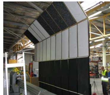
Fig. 6. General view of the acoustic partition wall in the workshop of aluminum pipe cutting
